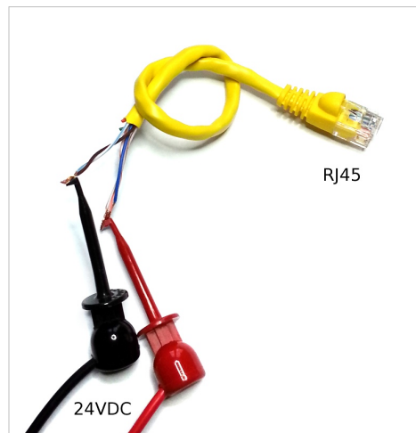
A quick'n'dirty way to make enable drive & disable safe torque off connection. May be used for testing before final wiring.
